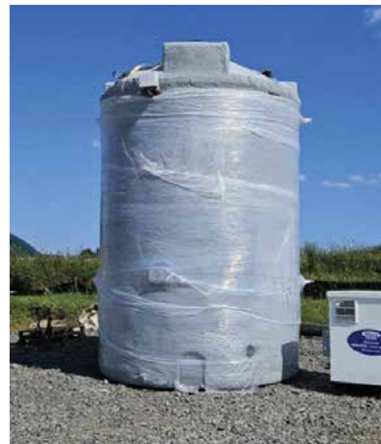
Chemical, Polyethylene tank
